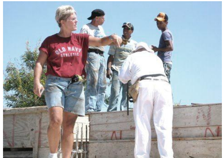
The 2010 Construction Team working on second floor roof with team leader Renee Liles
